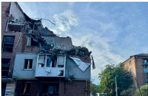
One of the Russian missiles hit a five-story residential building in Kharkiv, May 31, 2024. (Kharkiv Regional Prosecutor's Office)
