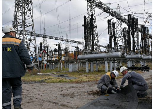
Energy workers of DTEK repair the equipment of power transmission lines, October 2022. Photo: Sergei Supinsky/AFP/Getty Images
